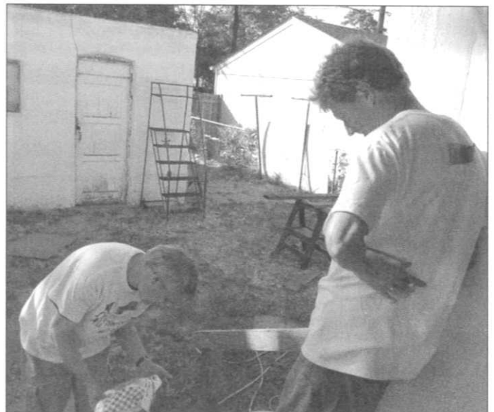
Doug Abbott and fellow Holland & Hart attorney Dennis Brown work on constructing and installing a hand rail attached to the back porch of the home.
